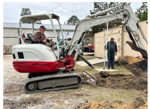
Jeffrey Ray & John Peck use a compact excavator provided by club friend Nick Brawn to prepare for pouring a flagpole pad and watch tower pad at the MVCSC compound. Thanks, guys!
